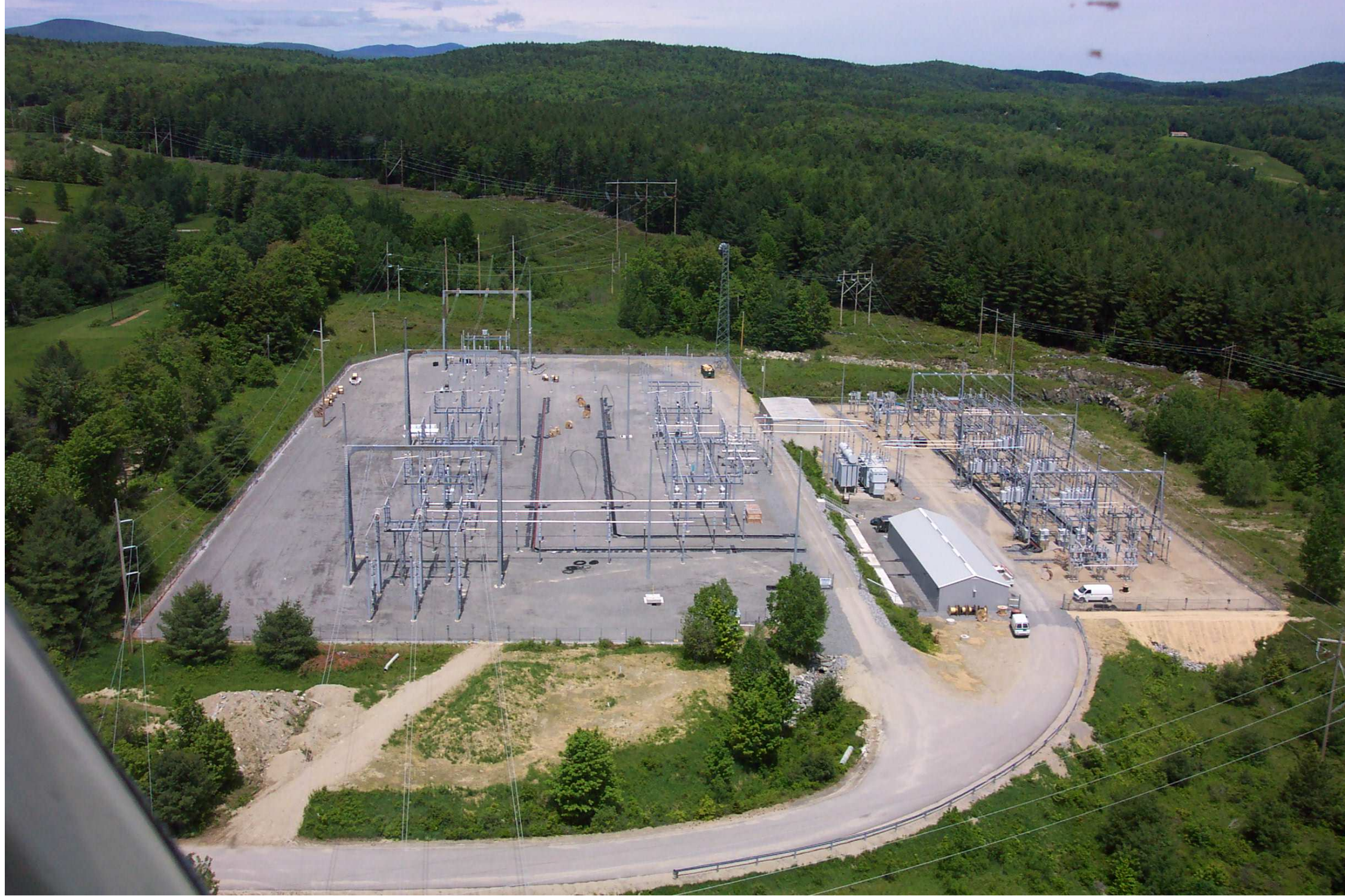
Coolidge Substation - Existing (2006)
