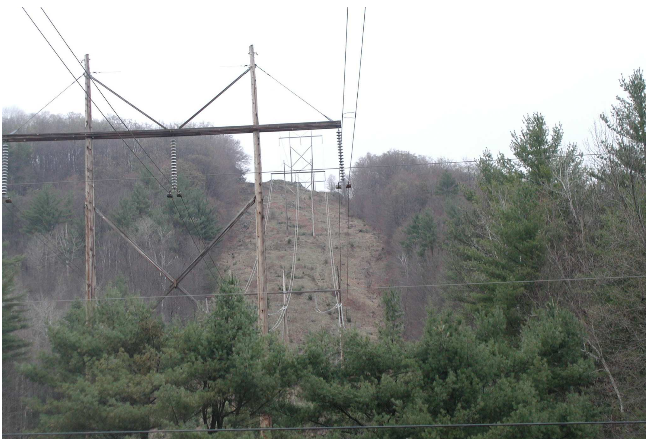
Coolidge to Vermont Yankee 345 kV Line (340 line) North of Route 103
